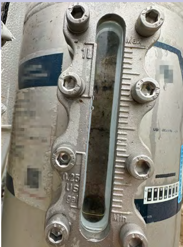
Empty pot showing leaking existing seal. The barrier fluid is leaking into the process due to inferior design.
