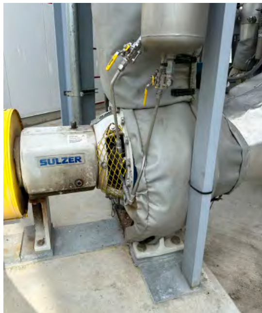
The pump installation with PPC seal (behind mesh screen).
